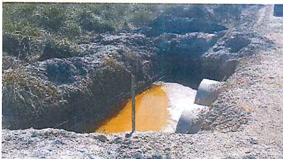
Figure 8: Culvert inlet after heavy rain - 25 October 2019
