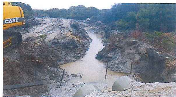
Figure 9: Culvert outlet after heavy rain – 25 October 2019
